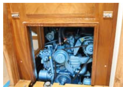
Forward access to the Nanni diesel engine
