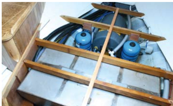
Fuel and calorifier tanks with the aft cabin berth being built around them
